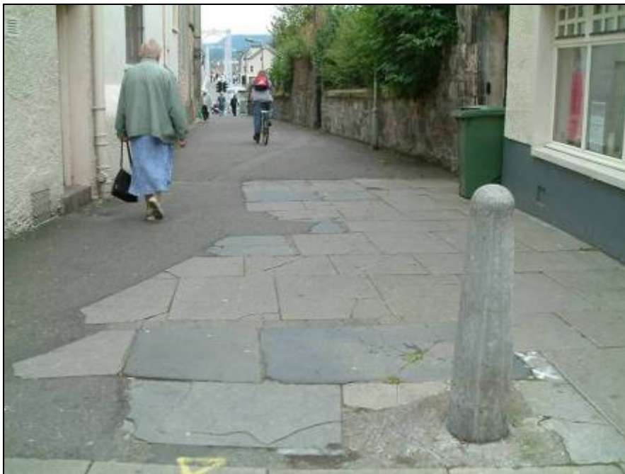
Figure 4: Before. Poor quality lane (materials, surface, obstructions)
