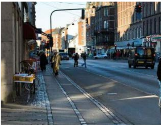
Completed footway, Vedbækgade, Copenhagen. Photo: Ramboll on behalf of the Road Directorate, Christoffer Askman
