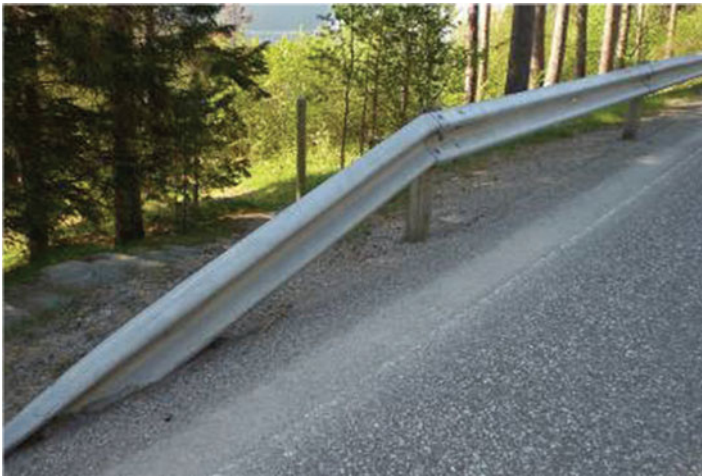
Fig. 4 Turned down guardrail terminal. (Photo: Marianne Gjerde (2008))
