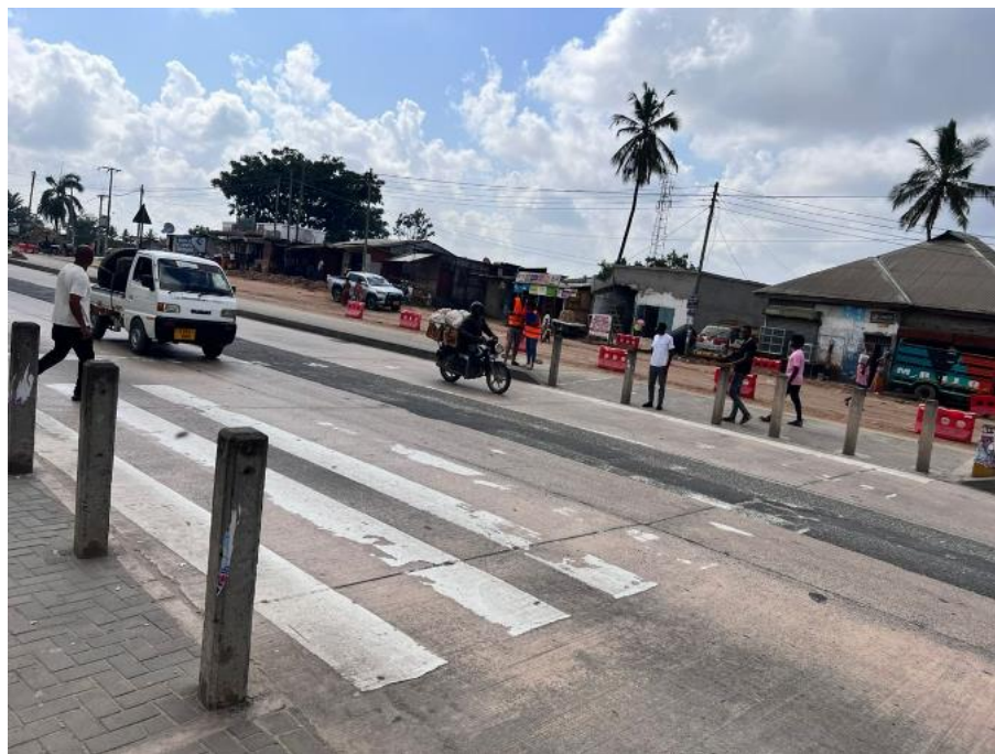
Figure 15. Worn crossing markings.
